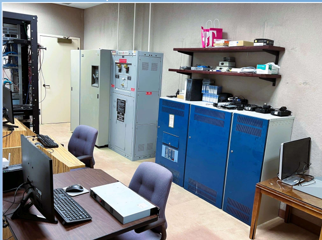
Raised Floor IT Room
