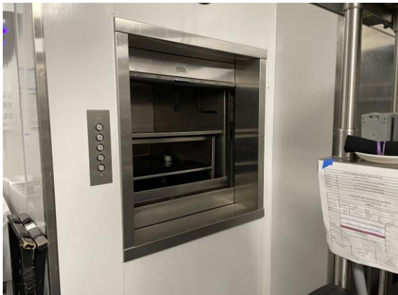
Dumbwaiter (1 st floor to 2 nd floor to roof top bar) Photo was taken November 22, 2023
