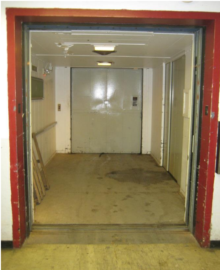
1 of 2 8-Ton Elevators Adjacent to Loading Dock
