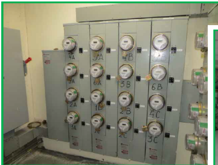
VIEW OF ELECTRICAL METERS
