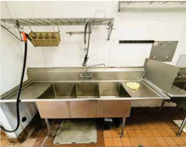
1795-#60 - In-Ground Grease Trap & Stainless Steel Sink
