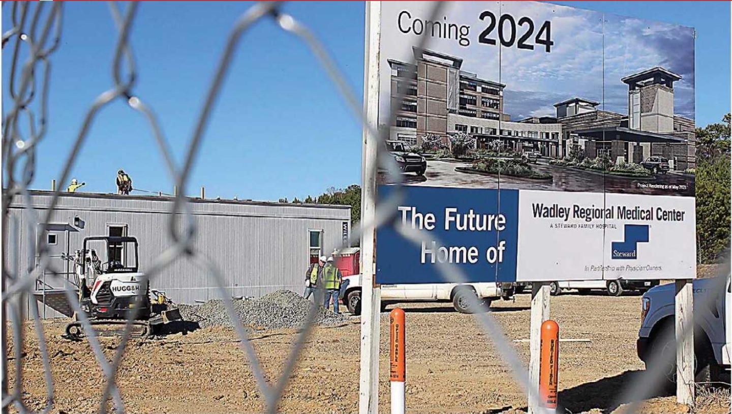
Workers erect office buildings for Robins & Morton at the construction site of Wadley Regional Medical Center on Friday afternoon in Texarkana, Texas. The project, at University Avenue and West Park Boulevard, is expected to be complete in 2024. The hospital will remain at its current location, 1000 Pine St., until construction is complete. (Staff photo by Stevon Gamble)
