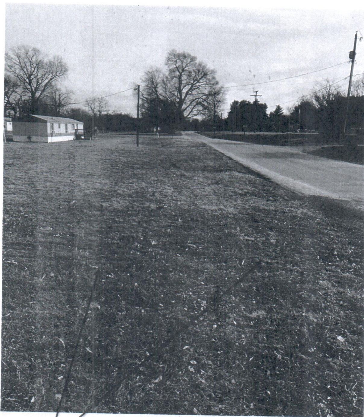
This image shows the two unknown utilities that are marked alongside the other road. The depths of these utilities is marked on the surface of the ground. It's tough to see the green paint but these two utilities run in a straight line alongside the road.
