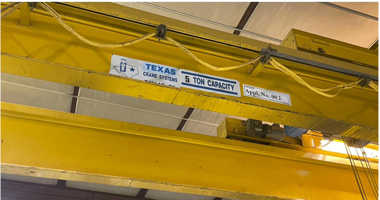
Main shop area has two, 5-Ton Overhead Cranes. Both span approximately 48 feet.
