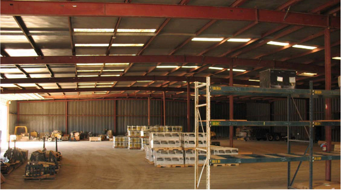
Warehouse has skylights and single bulb lighting. Opportunity to upgrade warehouse as needed.
