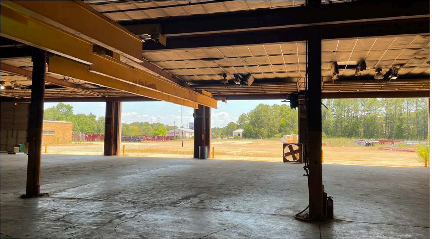
Main shop area looking out towards the south yard. View of two overhead bridge cranes.
