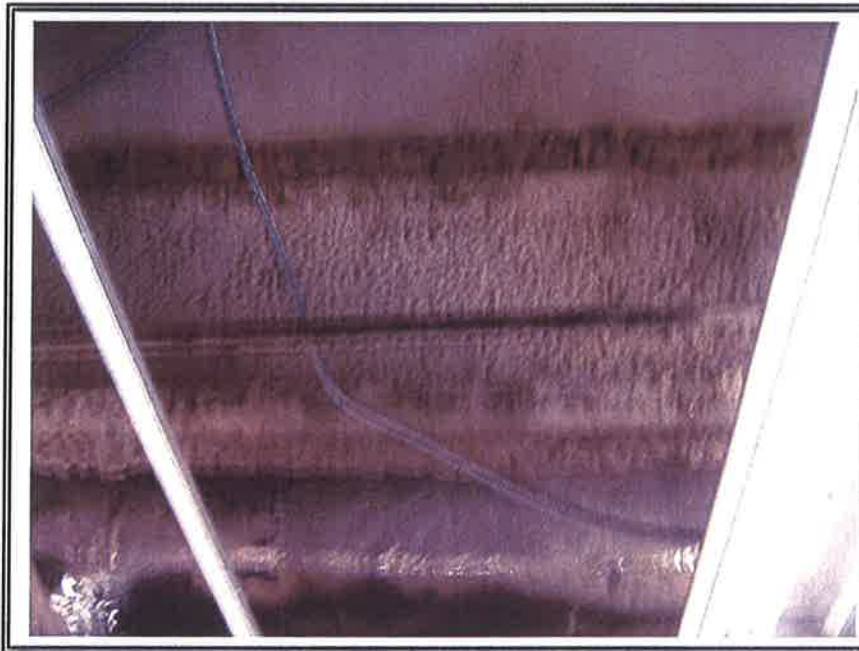
Photo No. 12: Photograph of fireproofing on structural supports located in the Main building.
