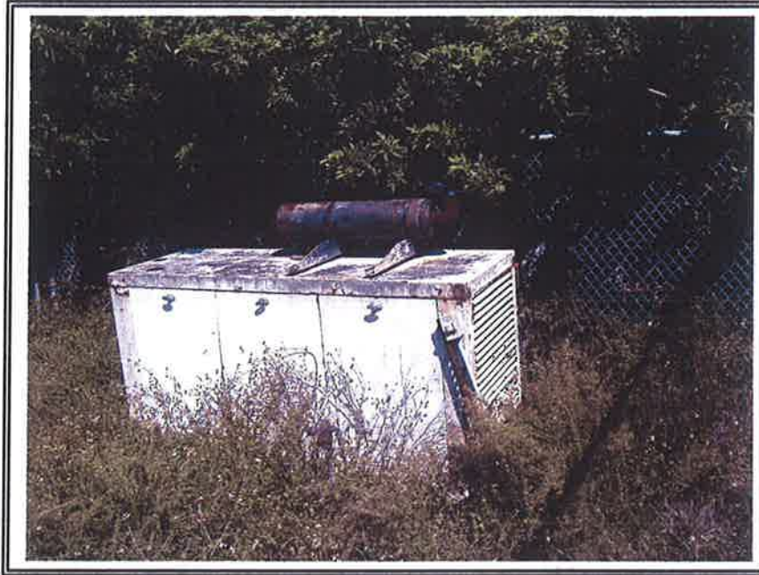
Photo No. 11: Photograph of generator located in a fenced area in the middle of the property.
