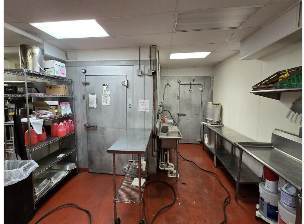
Walk-in refrigerator and freezer
