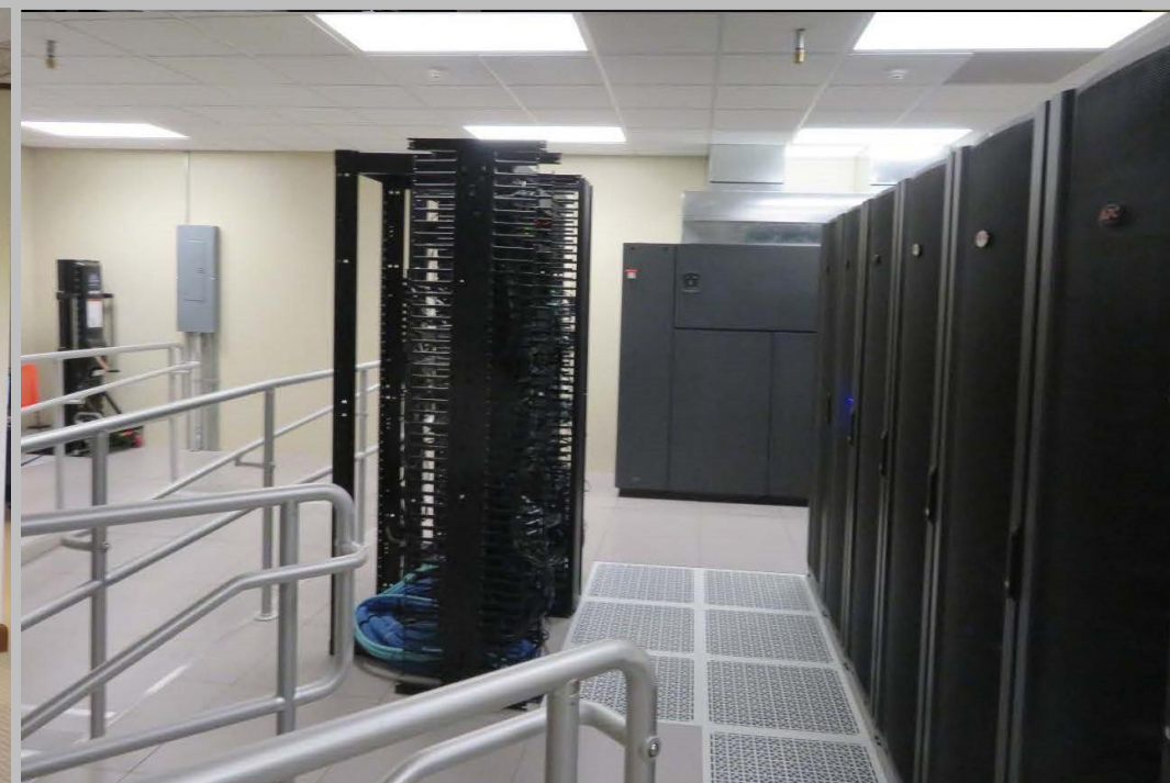
DEDICATED IT SERVER ROOM
