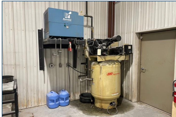
10 HP Air Compressor/Air Dryer
