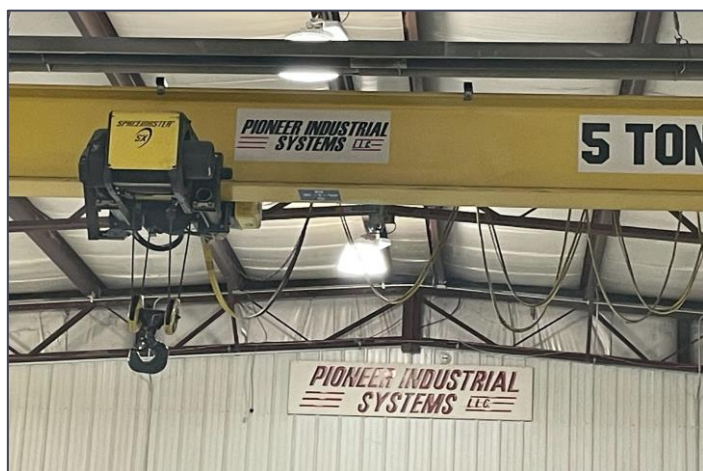
Overhead Crane – 5-ton/Overall 10-ton Capacity
