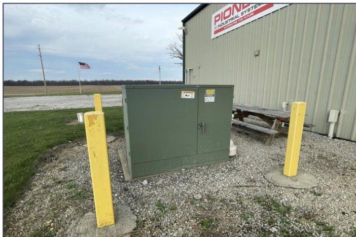
Transformer – 480V – 3 phase – 400 amps
