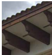
9 WOOD OUTRIGGERS BROWN TEAK WOOD REF. MATCH EXISTING SHIPPING CENTER REF. COLOR CUSTOM BROWN SEE 3/A-400
