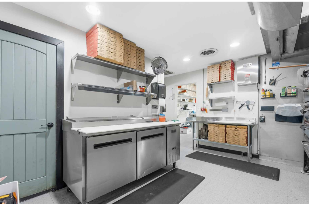
Restaurant Commercial Kitchen.
