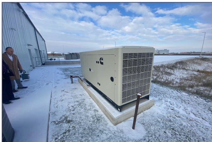
Natural Gas Generator
