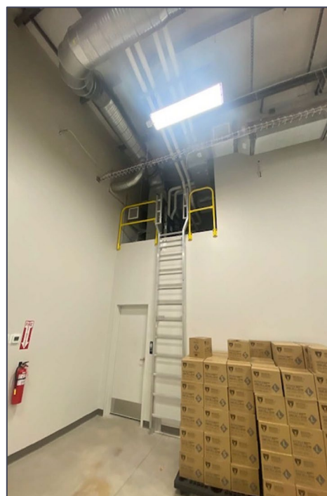
Access to HVAC
