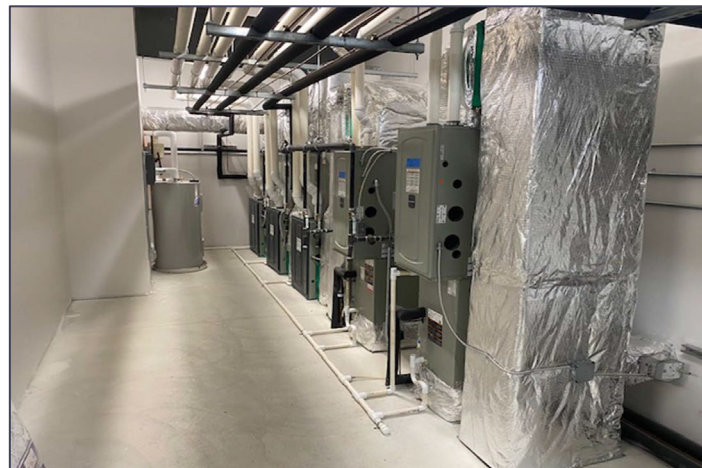
5 HVAC Units Above Office
