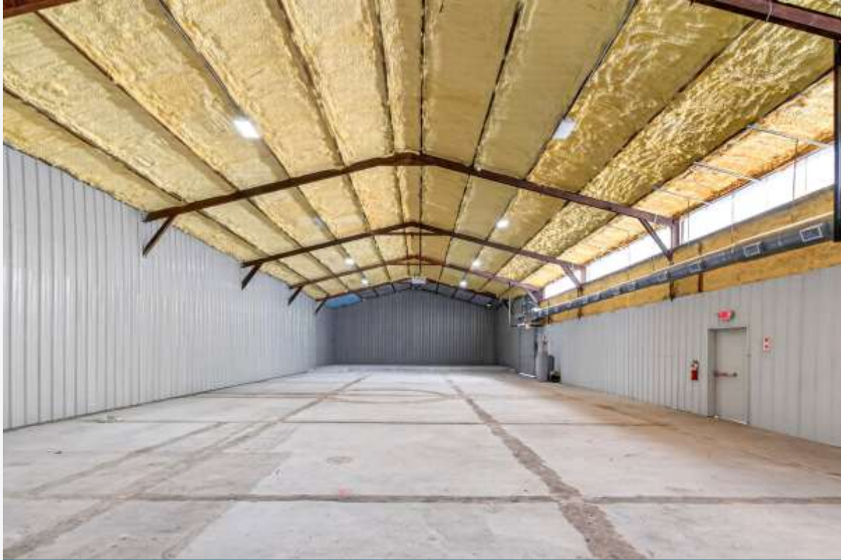
◆ FULLY A/C Building A — HVAC-Controlled Warehouse (±7,700 SF)
