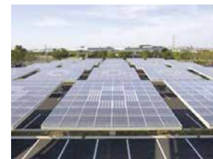
Photovoltaic panels on parking garages
