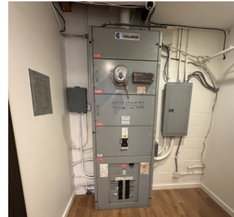
Main Panel is 400 amps and there are Two Sub Panels which are 200 amps each
