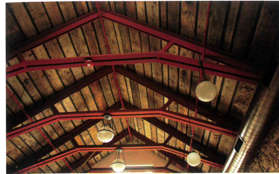
Most of the historic Firehouse's wooden ceiling boards were saved, refurbished, and reinstalled in the ceiling. (Photo by Eric Ming)
