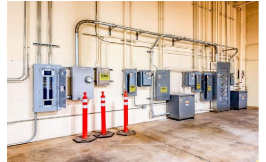
Electrical & power service
