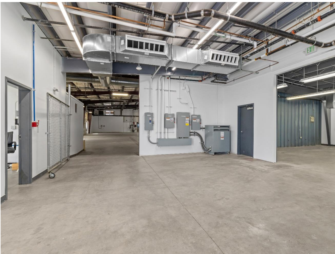
East end looking westward. LED lighting, heated/cooled make up and closed-circuit air supply ducts above.
