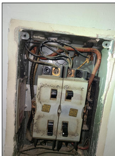
Old Electrical Panel
