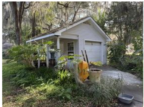
Exterior View of Outdoor Storage (Below Average Condition)
