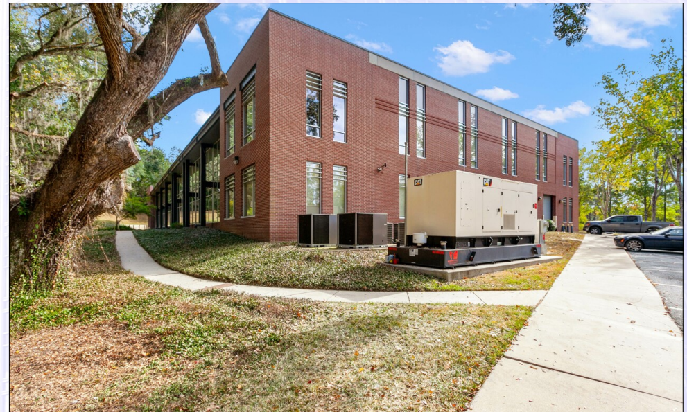
Full Building Generator-CAT 350KW
