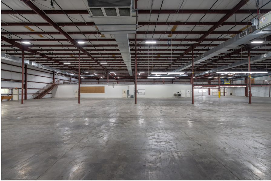
Warehouse Interior | 100% LED Lighting
