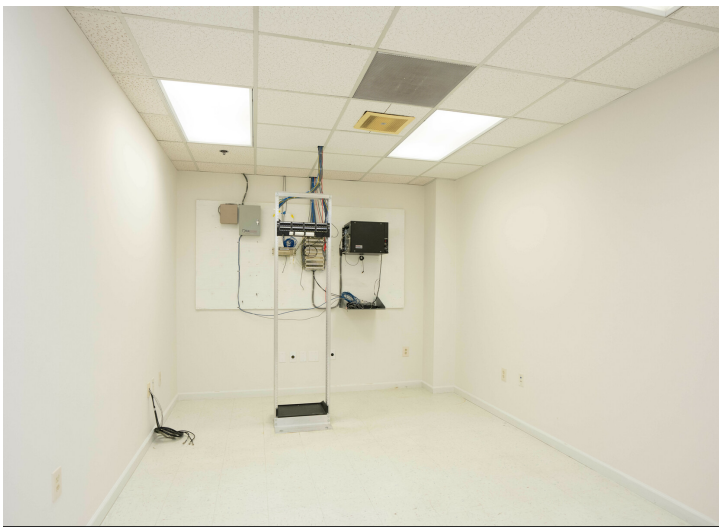
Dedicated Server Room
