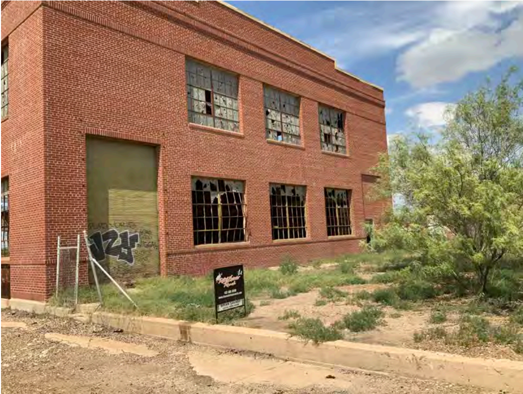
Site: 100 S. Elm Street, Pecos, Texas View of south side of subject and small lawn/yard area
