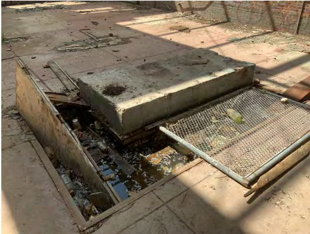
Looking at floor damage in west room
