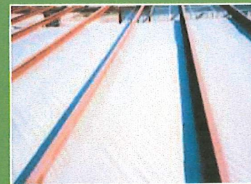
View of fabric liner positioned on strap platform and fastened to the structure.
