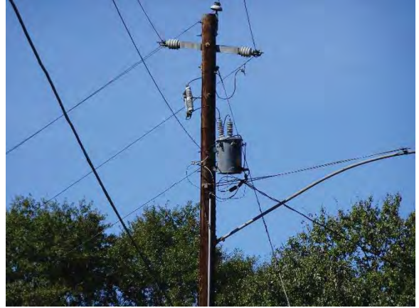
Transformer on Subject Property
