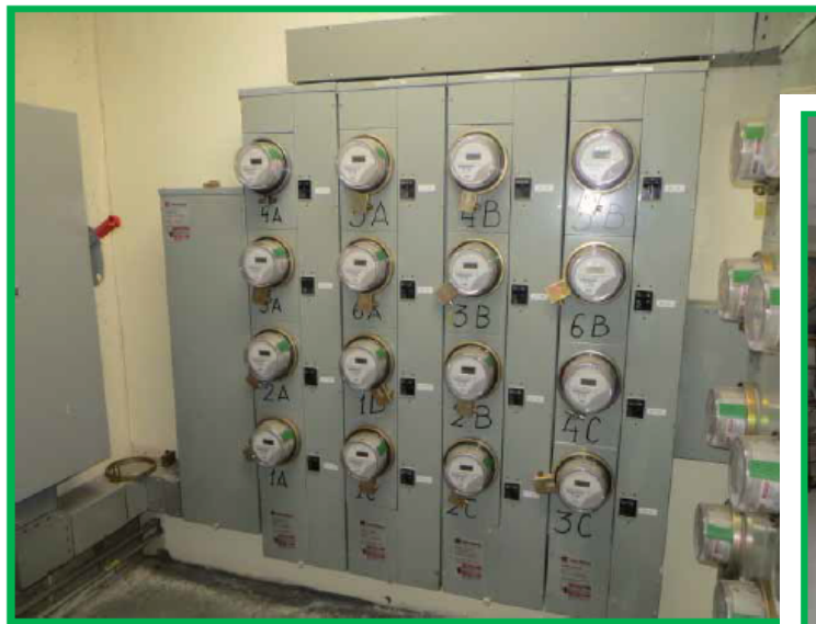
VIEW OF ELECTRICAL METERS
