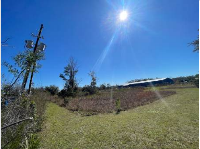
38. Pole Mounted Transformers
