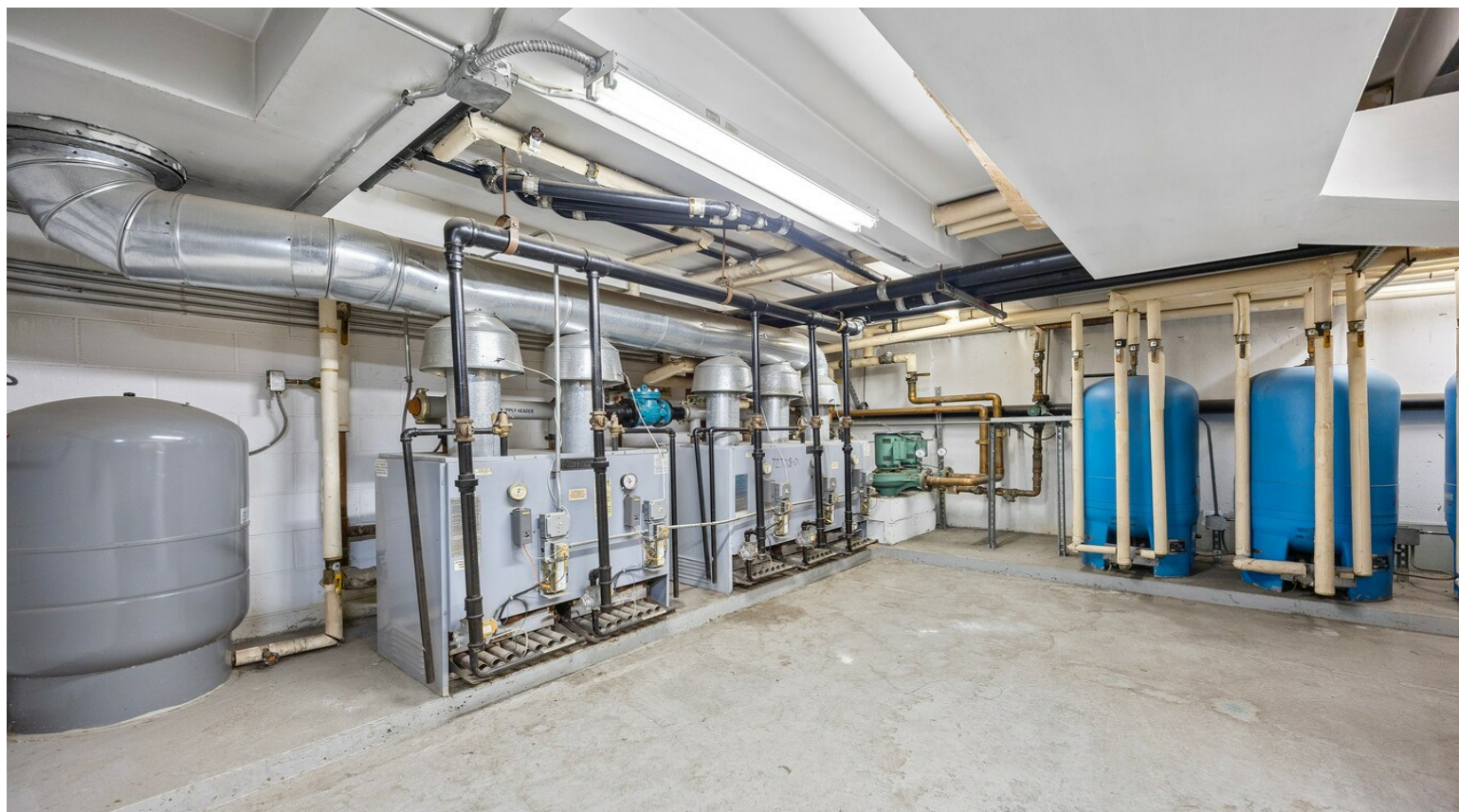
Gas, Multi-boiler Heating and Hot Water
