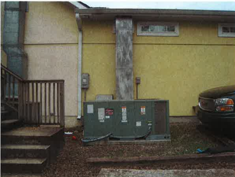
HVAC system unit serving the subject building.
