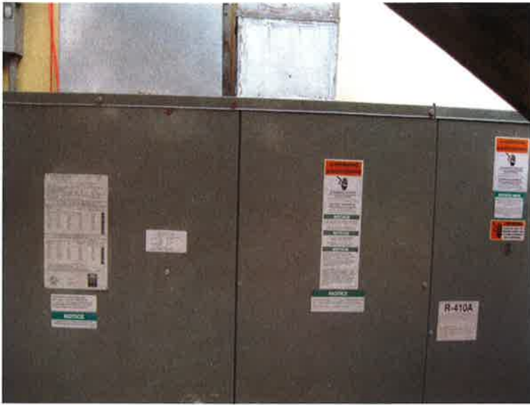
HVAC system unit serving the subject building.
