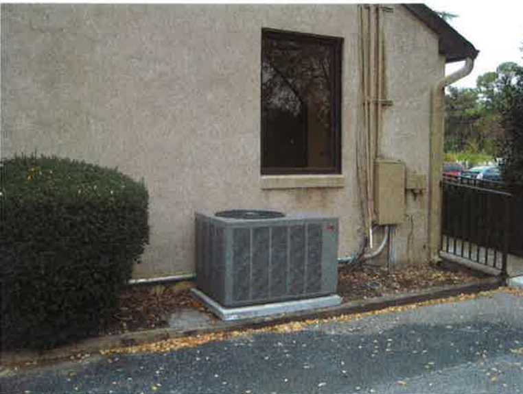
Central air unit.
