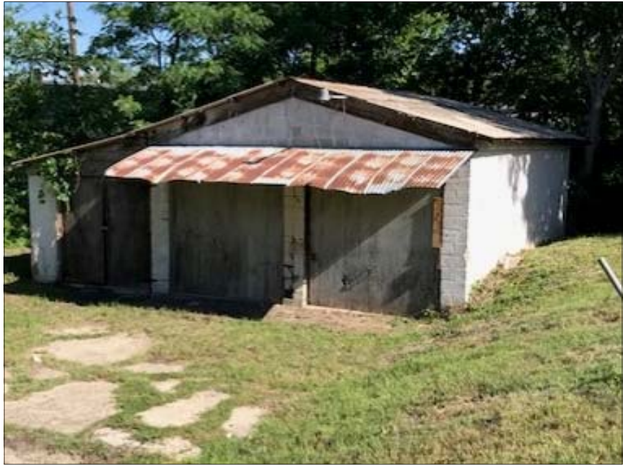
Photo 1: View of the garage located in the northwest portion of the Site, facing northwest.
