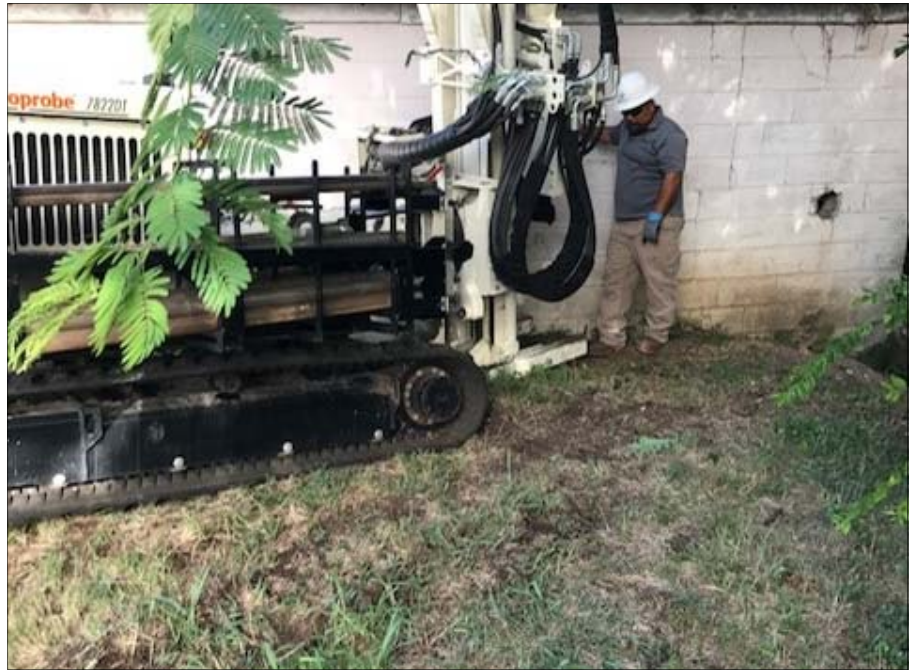
Photo 5: View of the advancement of soil boring B-7 located on the eastern exterior wall, facing west.
