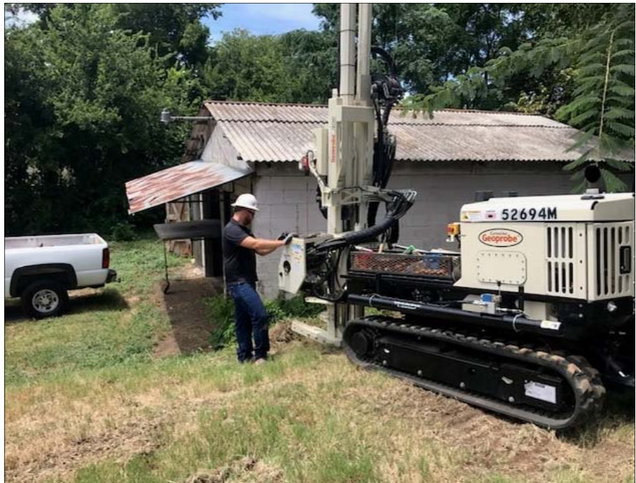
Photo 8: View of the advancement of soil boring B-10 located near the southeast corner of the garage building, facing west.
