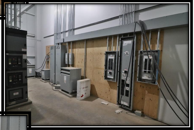
Electric Room- North
