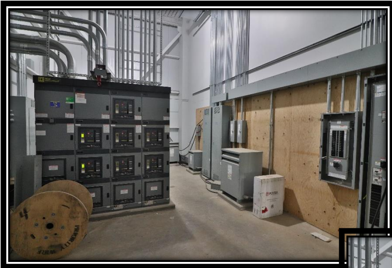
Electric Room- North
