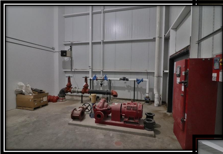
Fire Pump Room
