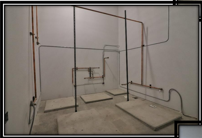
Air Compressor Room
