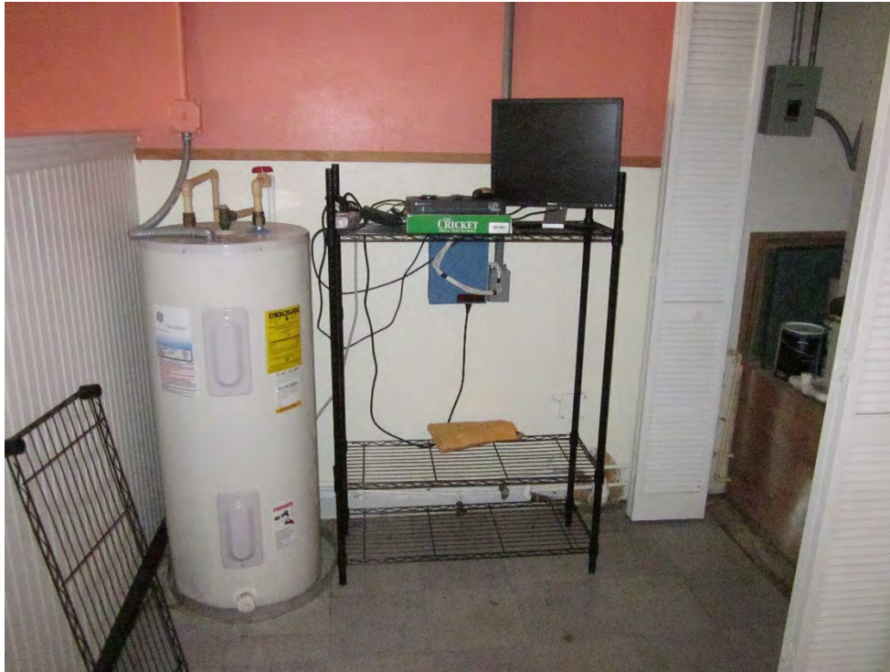
Site Photograph 29 – Water heater located in vacant lease space
