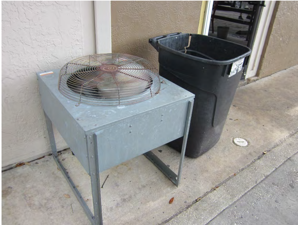
Site Photograph 35 – Cooling unit located at northeast corner of south Property building
