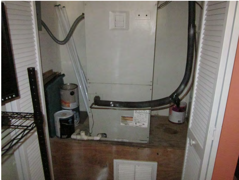
Site Photograph 30 – Air handler unit and spare paint located in vacant lease space
