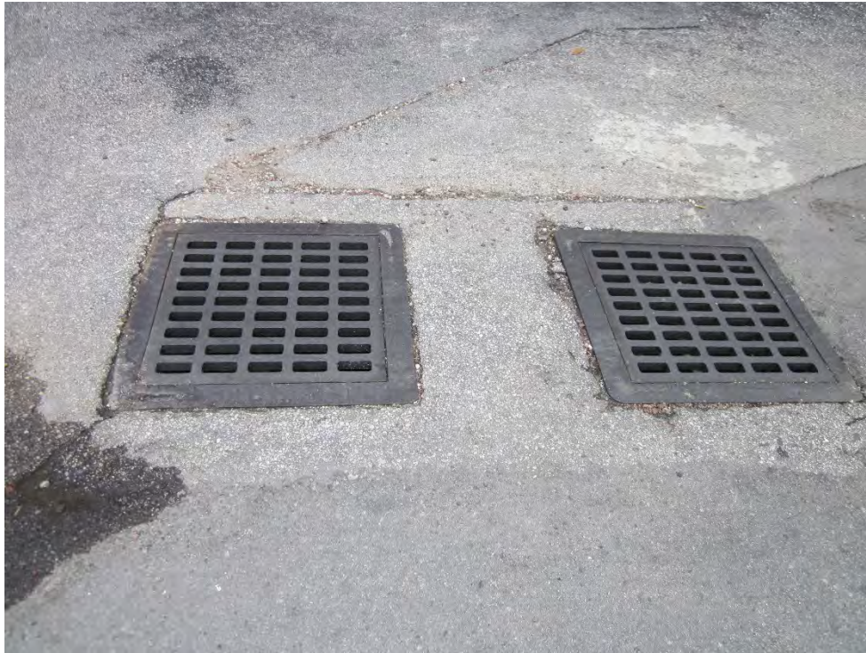
Site Photograph 41 – Storm water drains; west adjacent to northwest corner of south Property building
