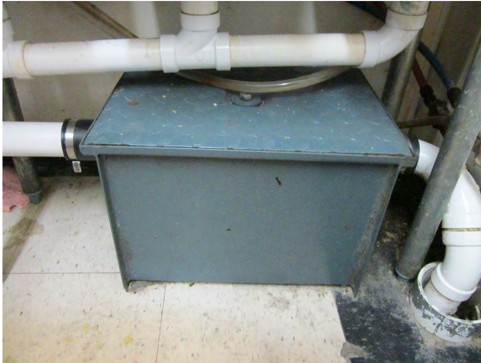
Site Photograph 17 – Grease trap located in the kitchen area of FFCB
