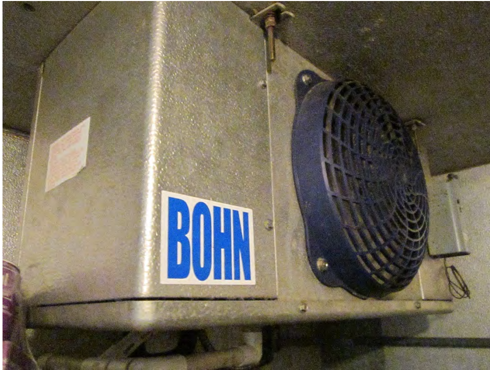
Site Photograph 19 – Cooling fan from cooler in Site Photograph 18
