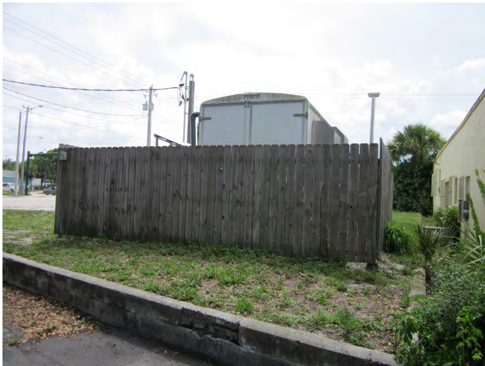
Site Photograph 44 – Remediation system located west adjacent to the southern portion of the Property
