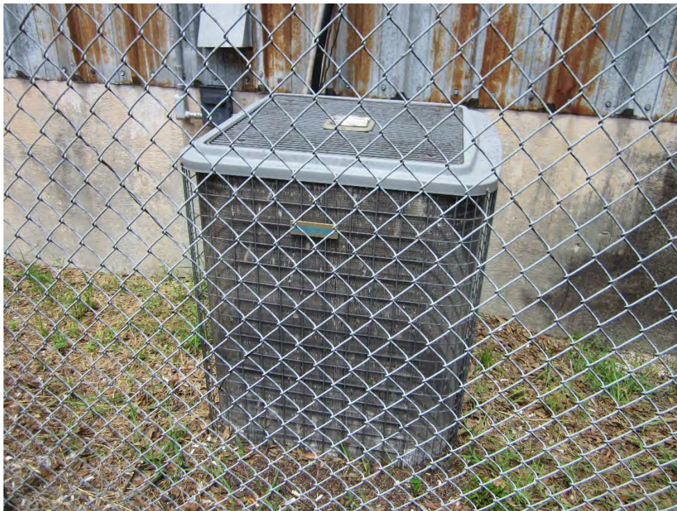
Site Photograph 46 – HVAC unit located on the east adjacent parcel
