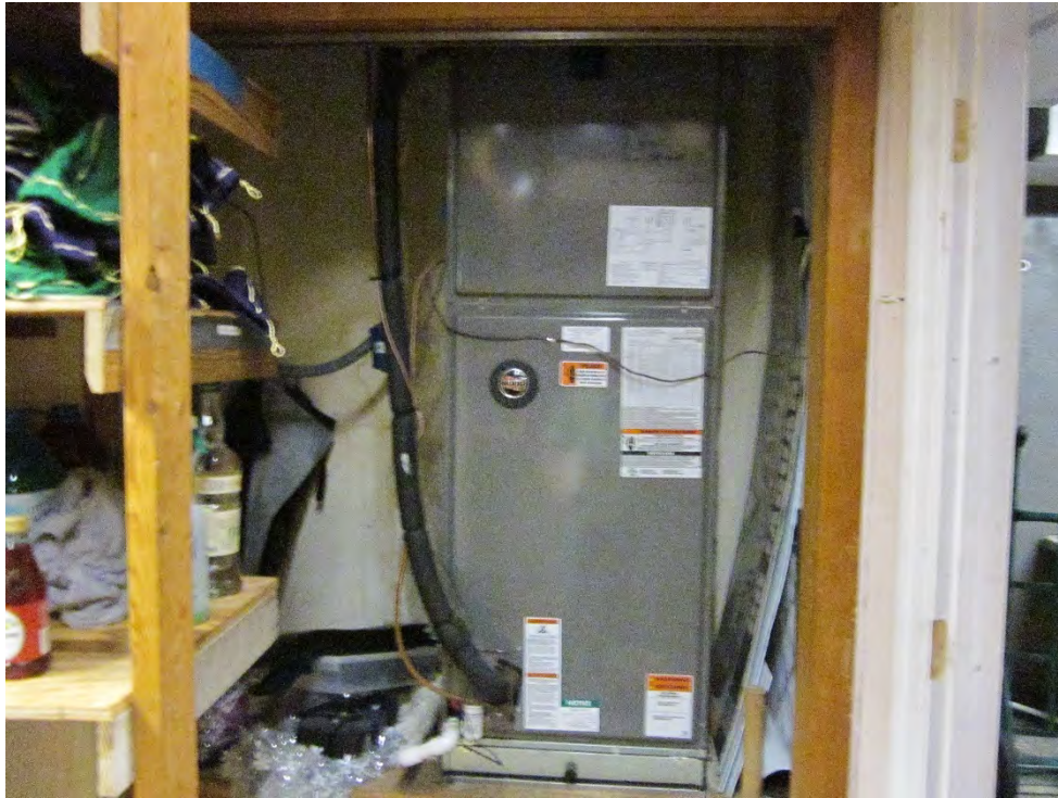
Site Photograph 23 – Air handler unit located in storage area of FFCB
