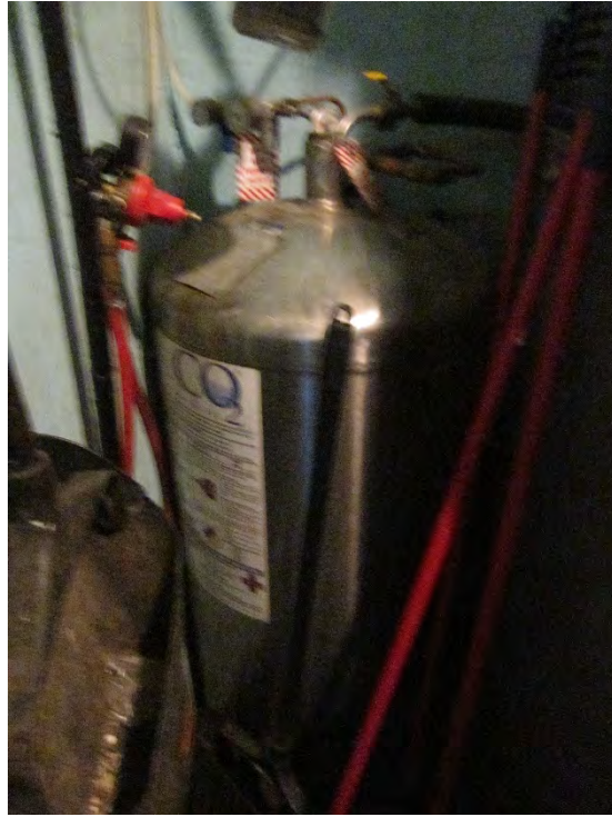
Site Photograph 15 – Compressed gas cylinder located in kitchen area of FFCB
