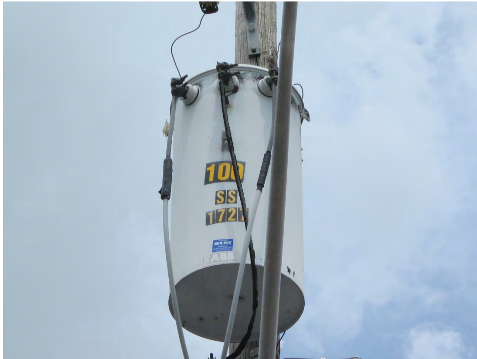
Site Photograph 40 – Closer look at transformer from Site Photograph 39
