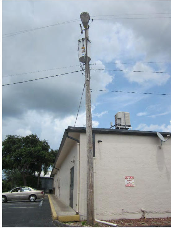
Site Photograph 39 – Pole-mounted transformer located at the northwest corner of south Property building
