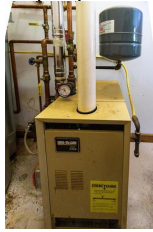
WEIL MCLANE BOILER for radiant heated floors
