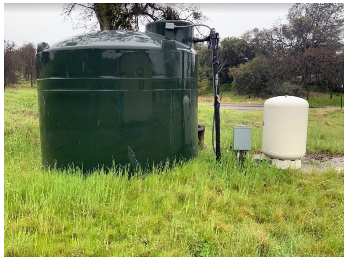
Well and water storage tank
