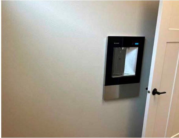
Water Bottle Filling Station
