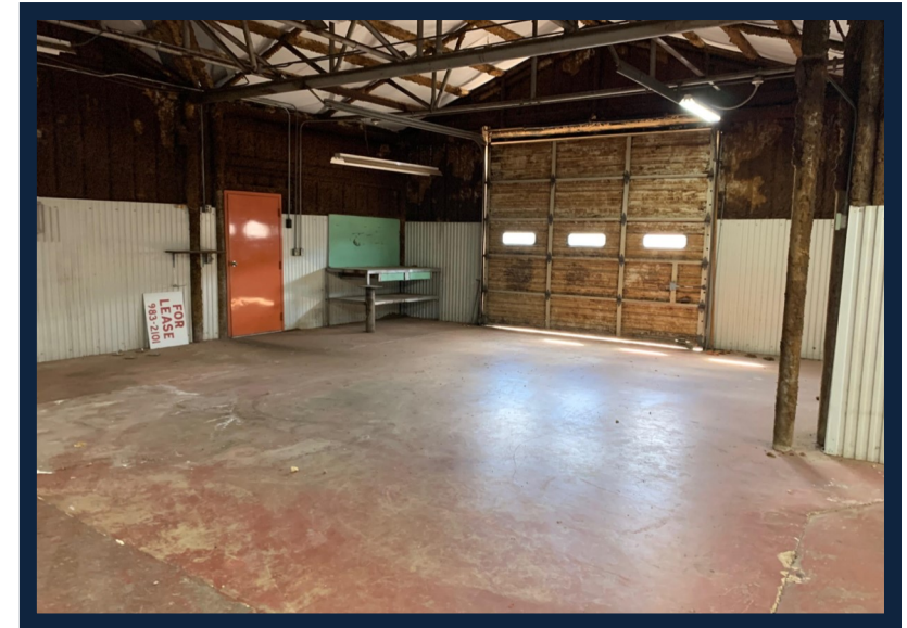
Shop Area with LED Lights
