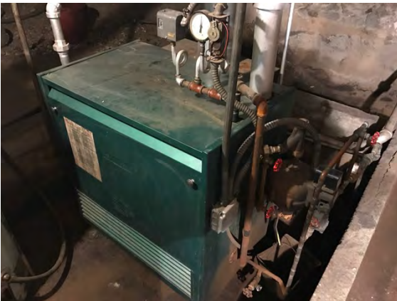
289 E 3 RD STREET GAS BOILER
