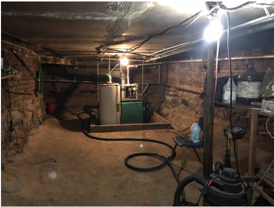
BASEMENT GAS BOILER & HW HEATER
