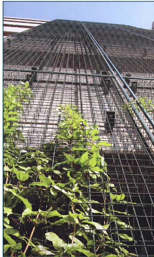
Green screen elements such as this wall-mounted trellis can act as heat shields and enhance the façade of a building.
