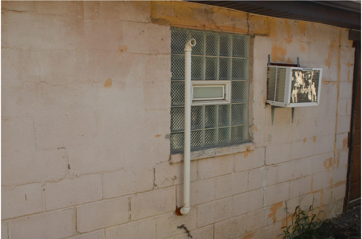
Improper plumbing vent in courtyard.
