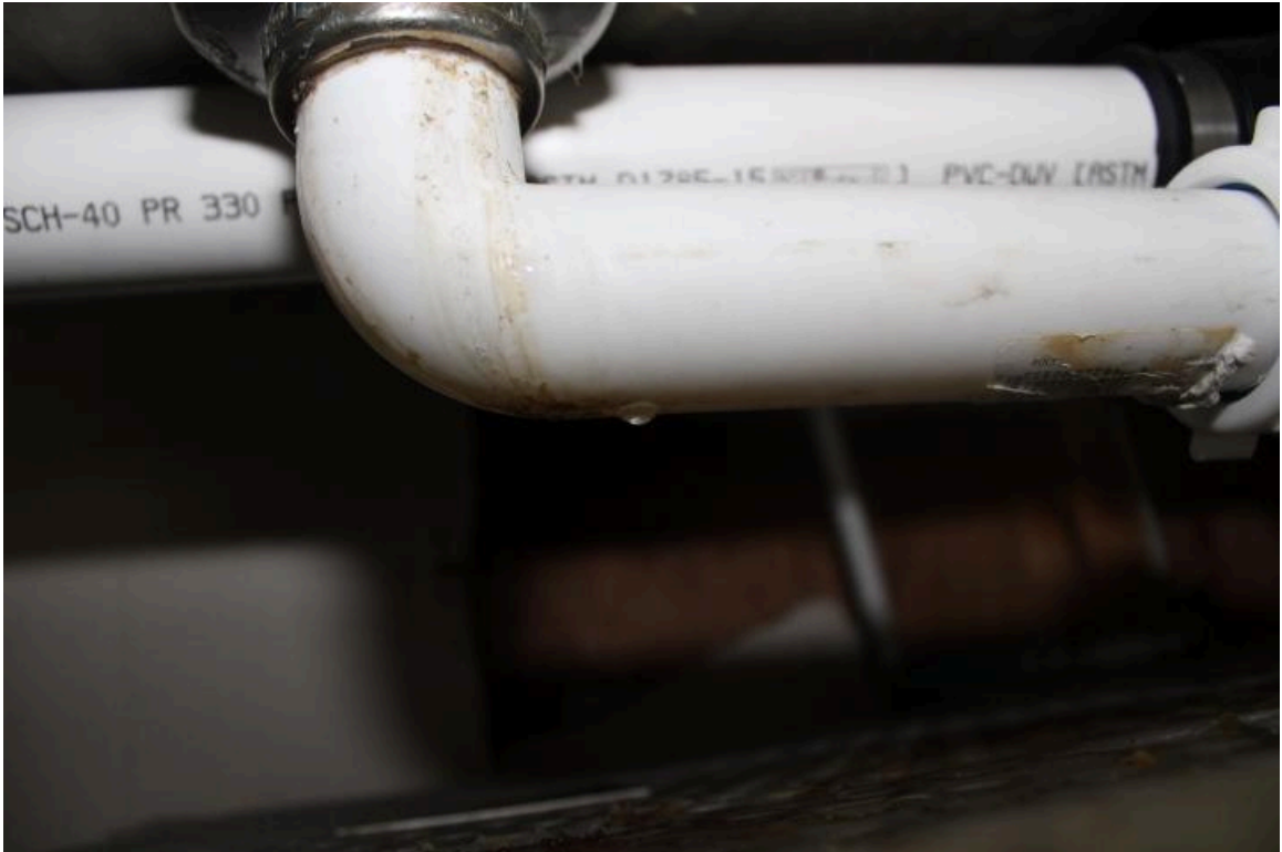
Leak on the kitchen sink drain.
