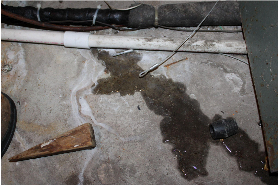
Unit #2 condensate drain line leak.
