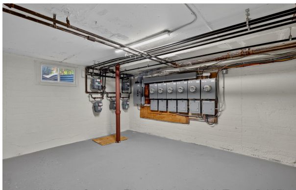
Basement Utilities — Separate Electric Meters per Unit (Tenant-Paid Electric)
