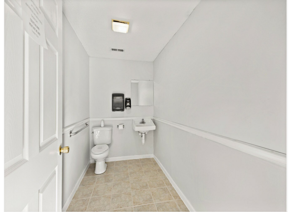
ADA Compliant Restroom 1
