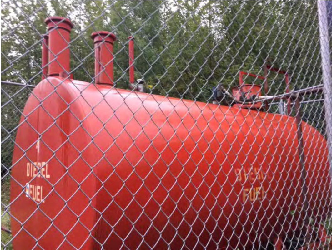
Photograph 13: 10,000-gallon diesel fuel AST
