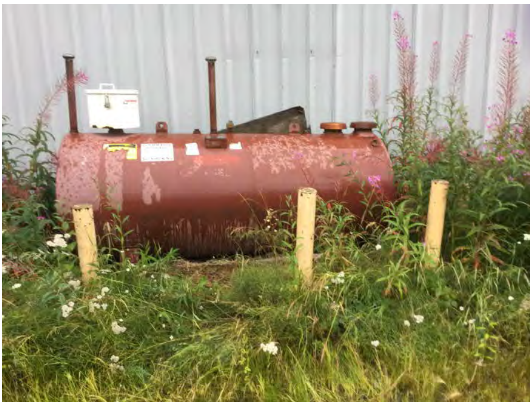
Photograph 15: Heating oil AST on building north side
