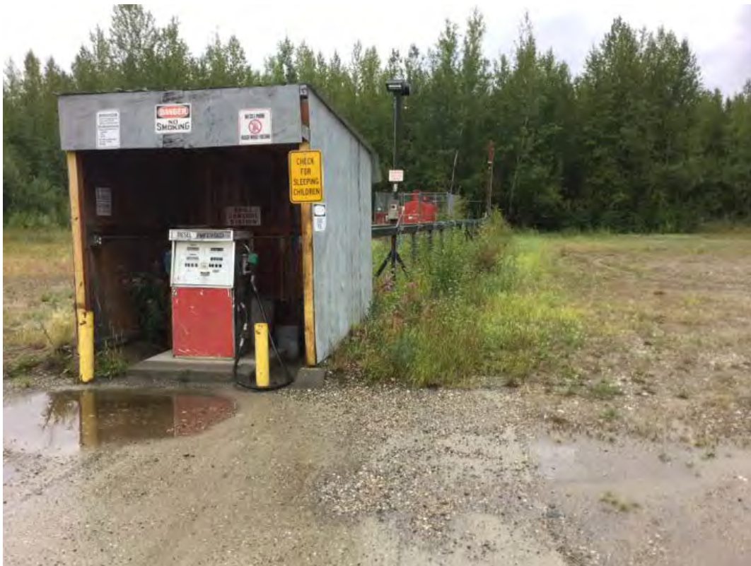
Photograph 14: Remote diesel fuel dispenser area
