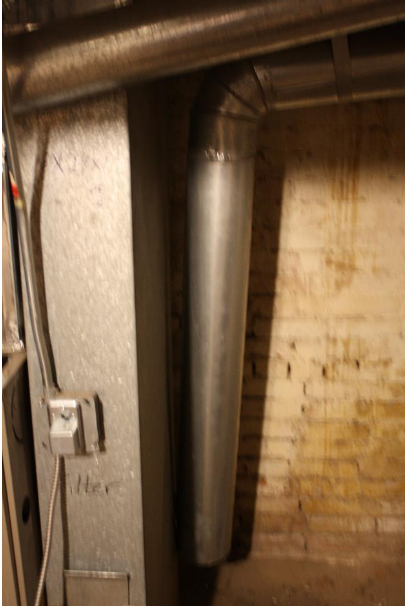
Hot Water Heater:
