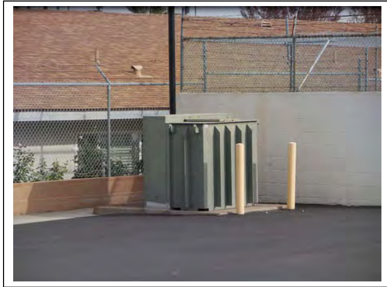
Picture (5). Pad-Mounted Electrical Transformer at the Subject Site
