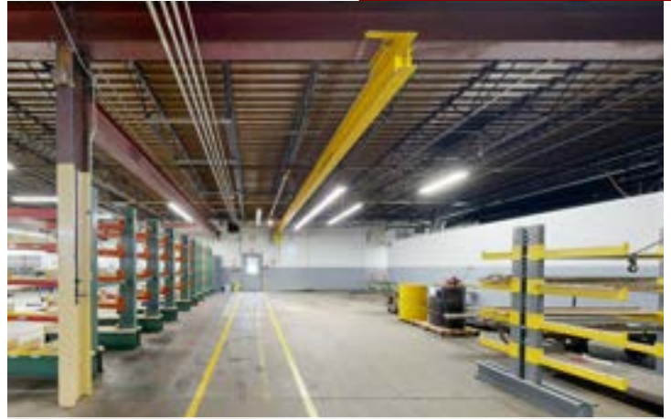
Half-Ton Monorail Crane - ±32'L Rail - 8'3" Under Hook (Bay 1)
