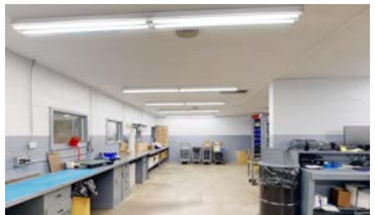
1 Of 2 Work Rooms - Additional Break Room, Locker Room, Utility Room, Restroom & 1,782± SF Mezzanine Above Work Rooms
