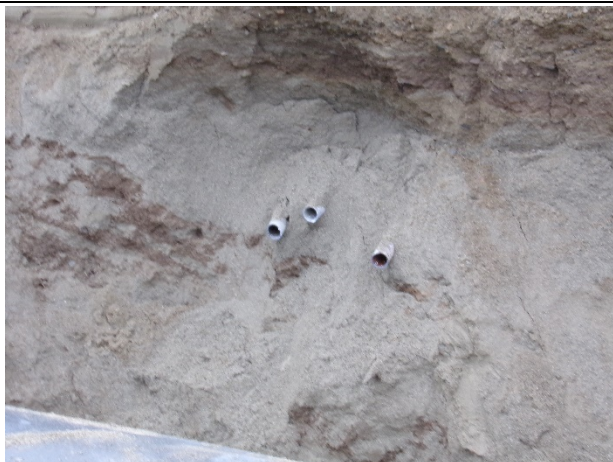
Photograph 11: Disconnected Fuel Lines
