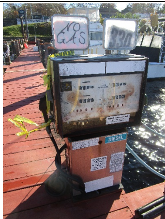
Photograph 3: Fuel Dispenser on Lower Portion of Site
