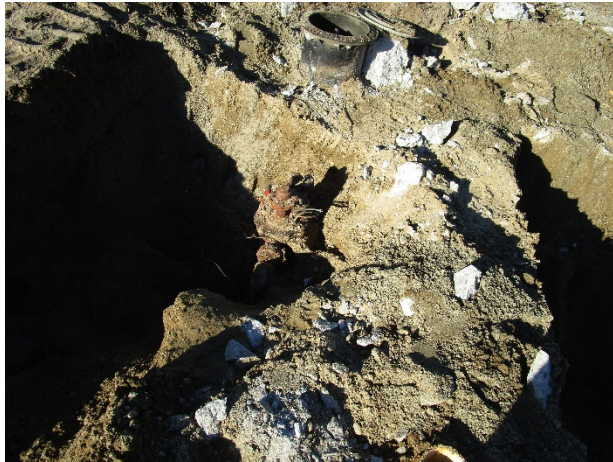
Photograph 7: Exposed Fuel Piping
